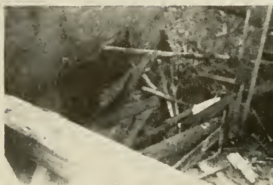
Debris in Front of the Penstock Gate
